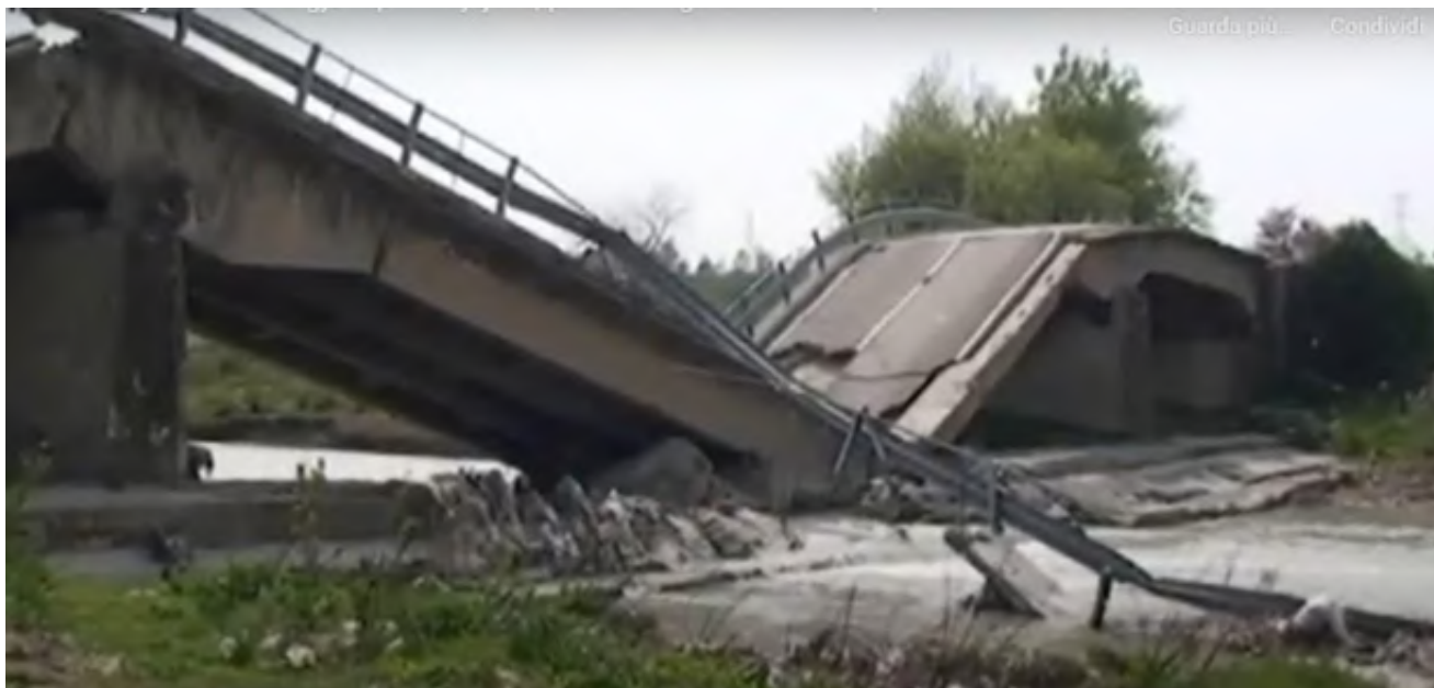
FIG. 1 – Typical damaged bridge due to the flooding.
