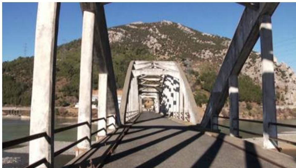
FIG. 4 The Zogu bridge, 2020- Some flooding caused erosion on the foundation piling, producing settlement
