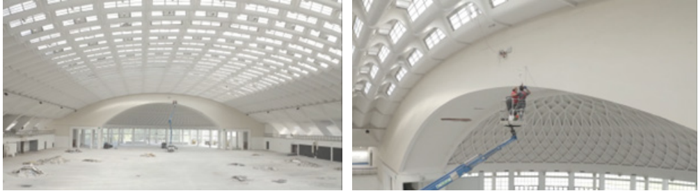
FIG. 19. – The inner part of huge barrel vault of Exposition Palace in Turin, by P.L.Nervi. On the right the moment of sensors installation
