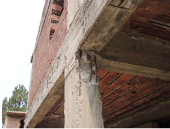
FIG.16 – The corrosion of the rebars in the concrete affect the quality of the material, and the resistance of the structural element can be much lower than what expected in the original design.
