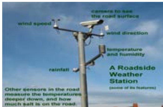
EXAMPLE OF A ROAD WEATHER MONITORING STATION
