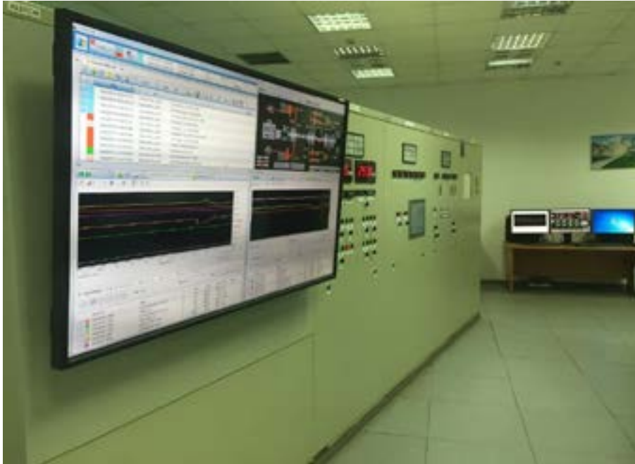
Figure 1: TPP Kosova B (digital monitoring of equipmentS)
