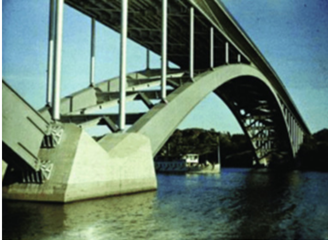
FIG.9 – The Västerbron bridge, in Stockolm, built on 1935, equipped with device within IoT platform (IoT Bridge-AB, Sweden, P. Rosegren,2017)
