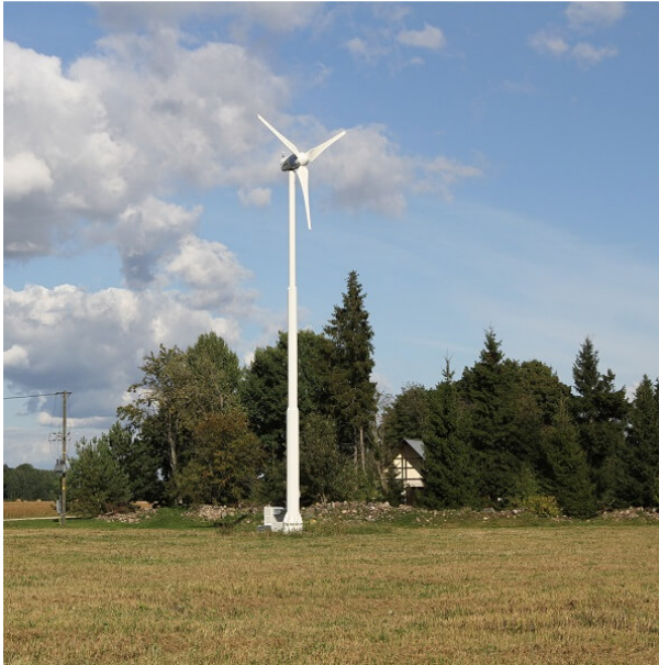
Figure 12. Illustrative photo, 10 kW wind turbine generator / Estonia
