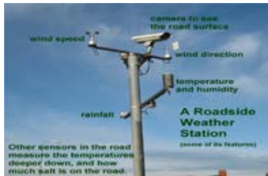
EXAMPLE OF A ROAD WEATHER MONITORING STATION
